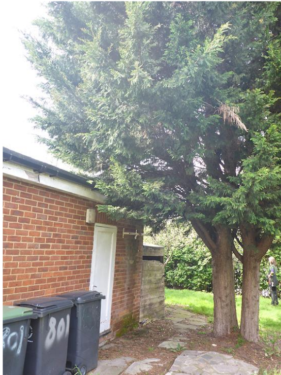
17. Leyland cypress: Crown lift to clear roof.
