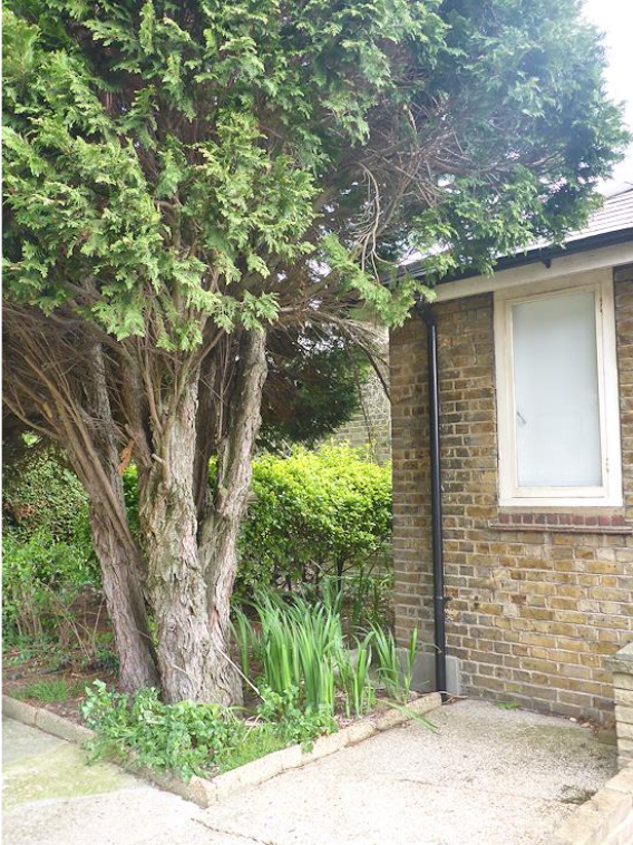
9. Cypress: Target prune to clear property by 1m. Cut wire embedded in trunk.
