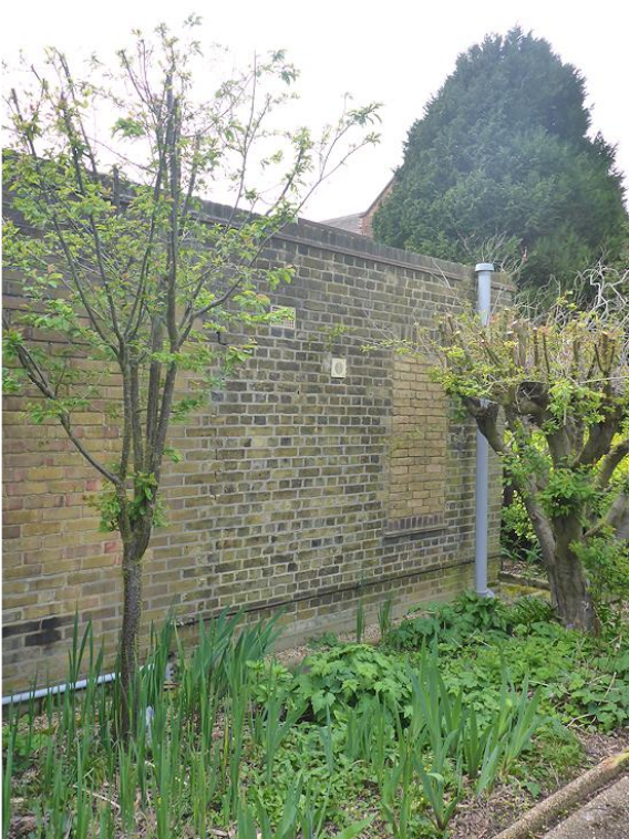
11. Chery x 2 heavily reduced. Very close to wall with cracks. Remove.
